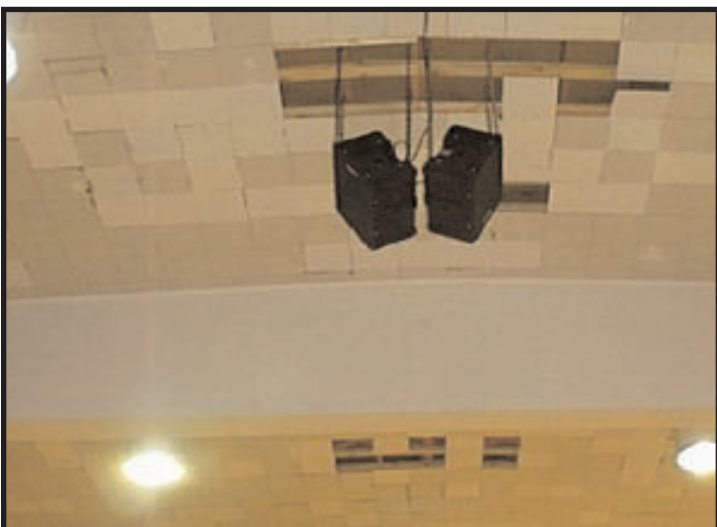
Turnkey PA System Installed in Gym
