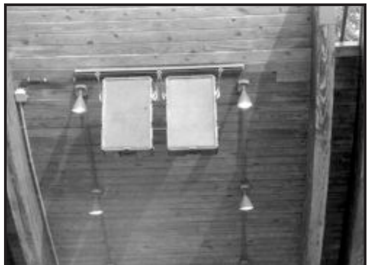
Turnkey PA System in Gym
